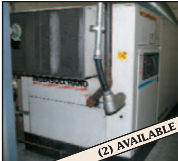
INGERSOLL RAND 150 HP rotary screw air compressor
