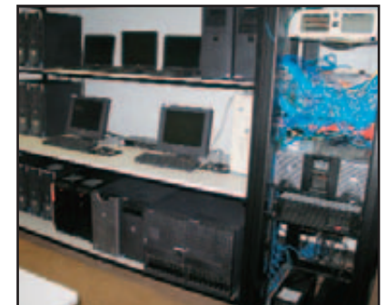
View of server room
