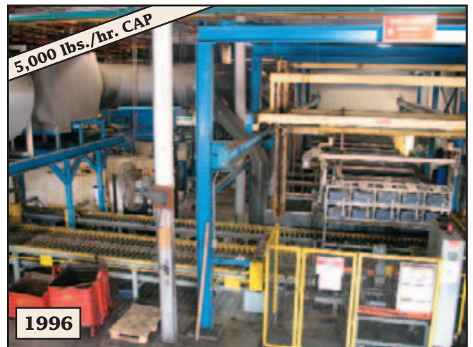
CEF Bright Dip Line & Water Treatment System
