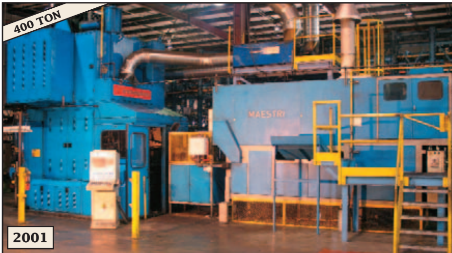
HYDROMEC HF 4000 CD hot brass forging press & MAESTRI TURBO GAS CT4-P 3500 4 track, gas fired, billet furnace
