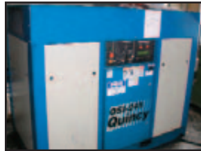
QUINCY 60 HP rotary screw air compressor
