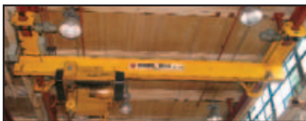
RICHARDS WILCOX 5 ton crane
